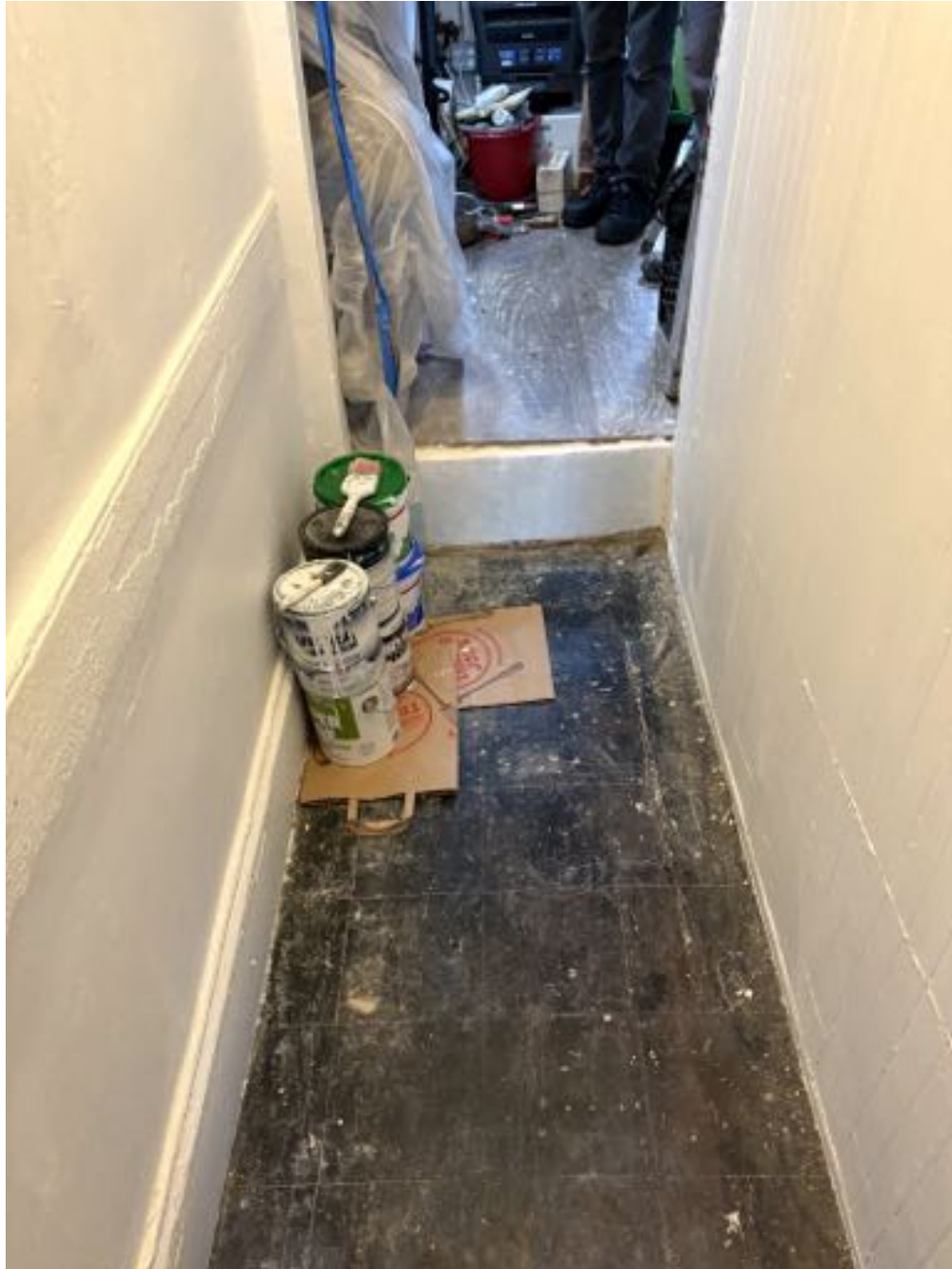
Figure 11: The entrance hall of unit 3D as observed on November 7, 2025. Note the slope of the hallway floor compared to the built-up leveled platform for the room beyond.
