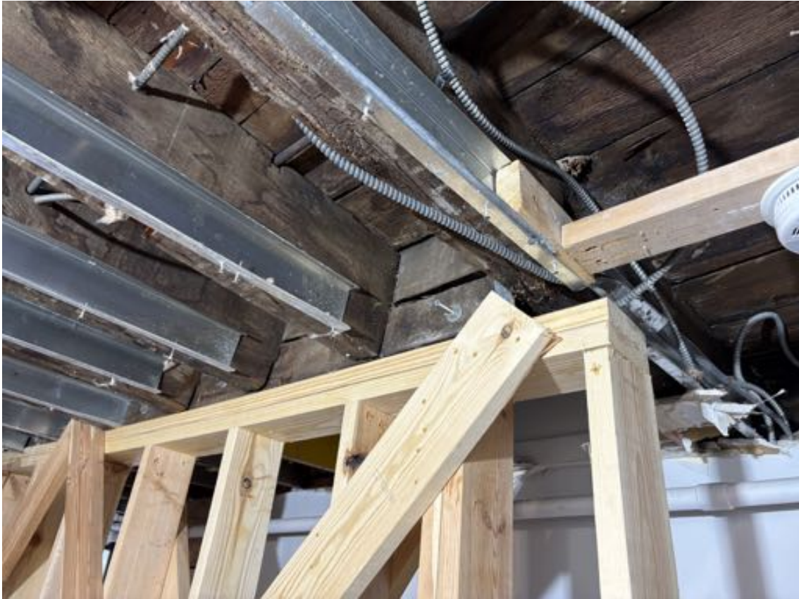
Figure 14: The header below the eastern stair bearing partition, as observed on November 7, 2025 in unit 1A. The light-colored wood is the shoring recently installed, and the crack in the header is visible at roughly the mid-height of the header and supported joists. The steel framing appears to be leveling for a ceiling that was not installed.
