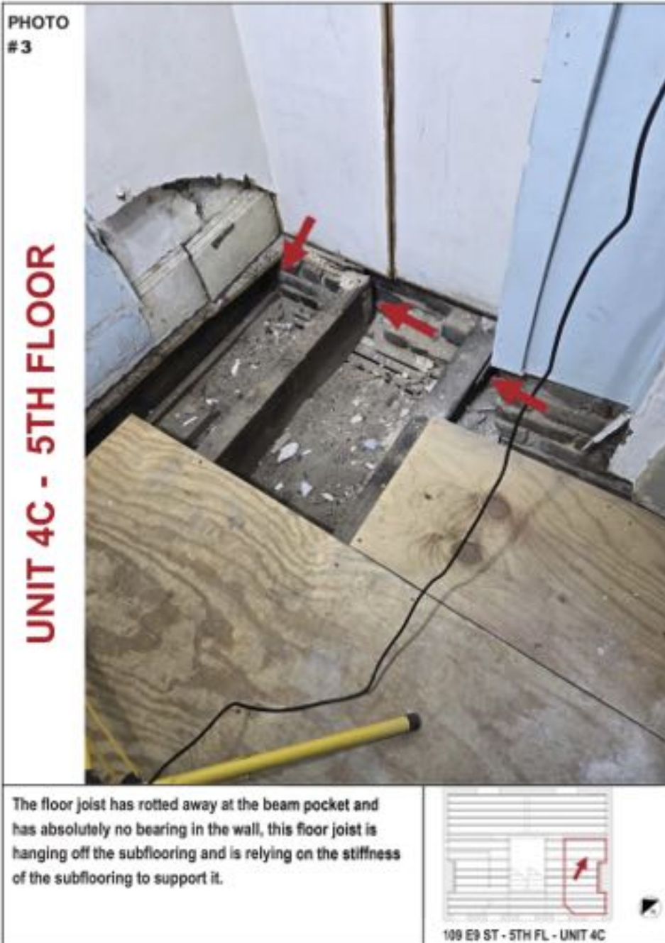
Figure 13: Photo 3 from the November 14, 2025 report by Steel Core Engineering. The red arrows are Steel Core annotation. The joist ends are damaged, but the joists extend into the brick wall and therefore have bearing and the rightmost joist has a wall tie (visible immediately to the left of the rightmost red arrow). The mortar is deteriorated but the wall is in position.
