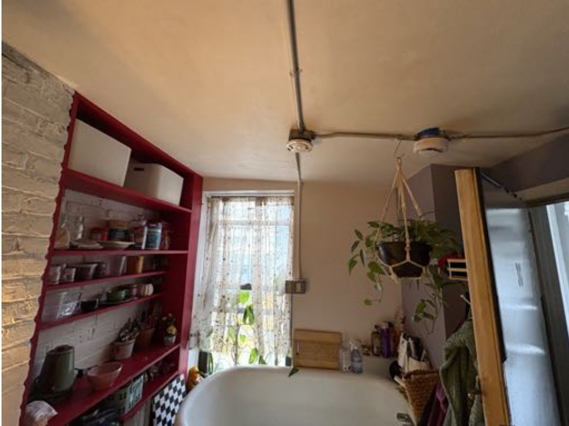
Figure 15: Interior of unit 3C as observed on November 7, 2025. Note the slope of the ceiling, following the slope of the floor above. The lack of plaster damage where the ceiling meets the wall indicates that this is not recent movement.
